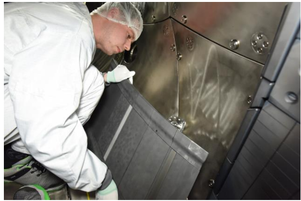
Fig. 5: Fitting the first wall into the bearings on the base plate. Repetition accuracy for re-installation are only some tenth of a millimeter. No further alignment is necessary.
