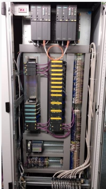
Figure 2: Redundant safety PLC (top) and Profibus-Safe fibre ring lines
