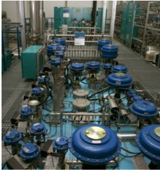
Fig. 2. View of cold box
