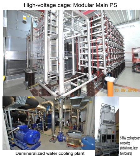
Figure 6. Key components of FULGOR test stand at KIT. Top: high-voltage cage with the modular main power supply. Bottom, left: demineralized water cooling plant. Bottom, right: 5 MW cooling tower on rooftop (currently one, later two towers).
