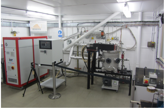
(b) (from left to right) water supply, induction heating, vacuum vessel, and control cubicle
