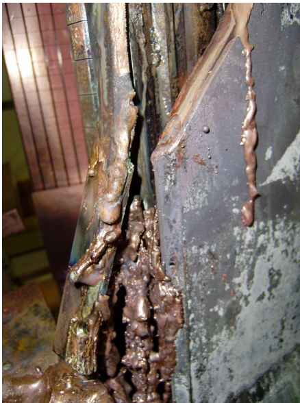
Fig. 3. Melt damage of a calorimeter panel
