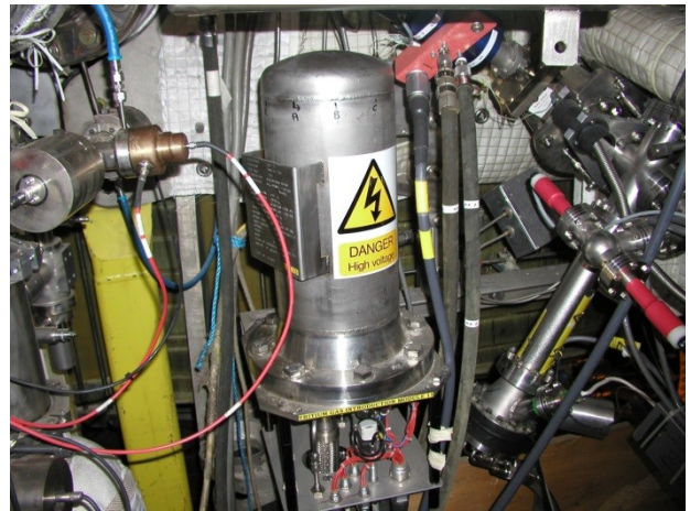
Fig. 1. GIM 15, the tritium delivery module for the DTE1 campaign (to be replaced by the TIMs).
