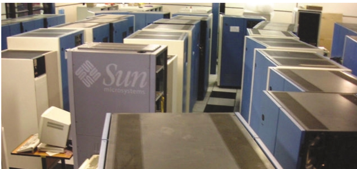
Figure 4.7: Sun equipment. Space was always a problem during campaigns C1-C4
