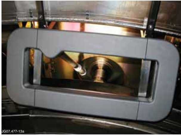
Figure 13a: One of the new active MAST AE antennas, as installed in-vessel.
