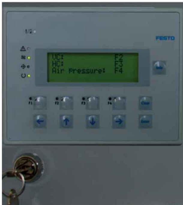
Figure 4: PLC Cubicle-Operator unit interface.
