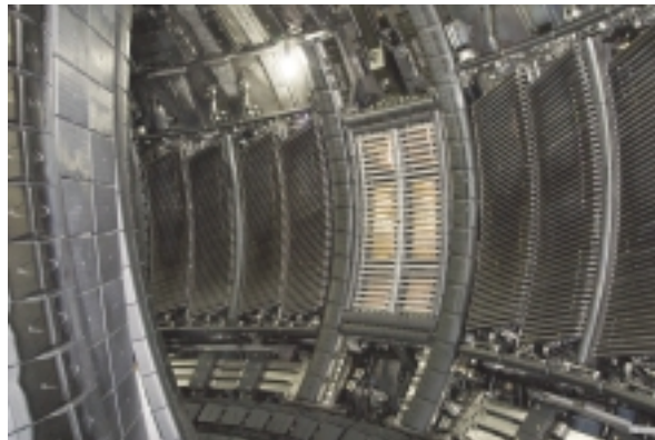
Figure 4: The ILA installed on JET between A2 antenna arrays A and B. The surface of the ILA aiming at coupling 7.2MW with a power density of \sim 8\text{MW/m}^2 is less than half of that of one A2 array.
