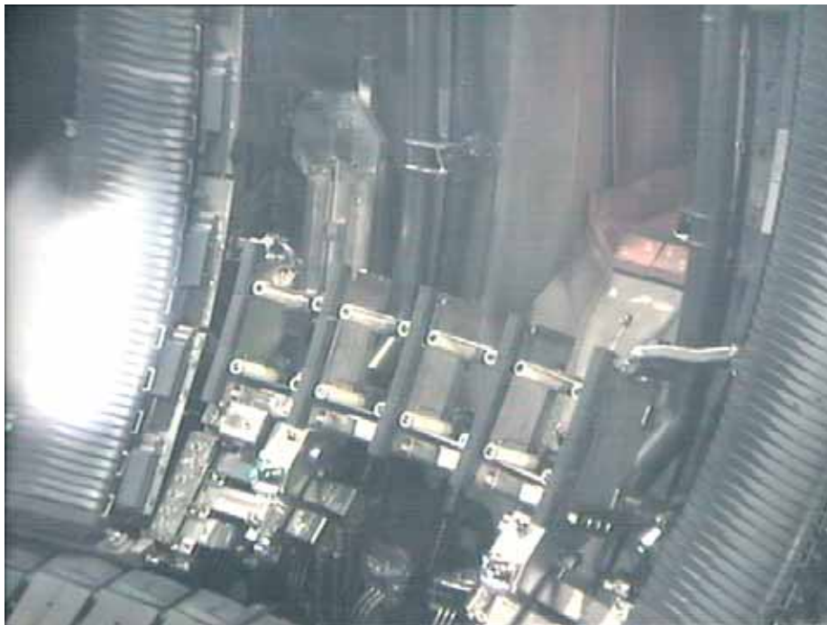
Figure 1. View of one group of four AE antennas as installed in vessel during June 2005.
