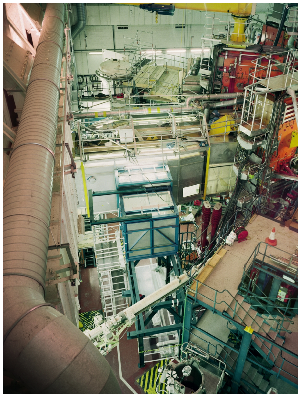
Figure 5: Ventilation system on Boom Enclosure
