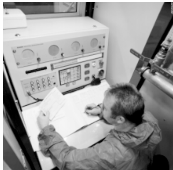
Fig.4: CDU control station.
